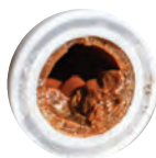
Blocked valves and pipes.
